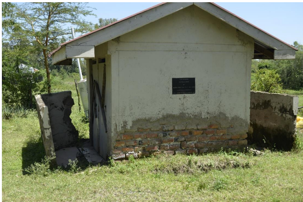
Closed toilets rendered unsafe to use because of sinking ground.
